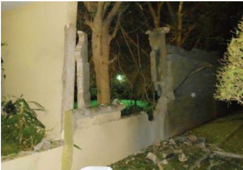
Damage at the Compound from an explosive device on June 6, 2012. (State Department photo)
